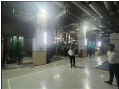
View of DG Room
